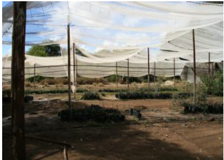
Mapungubwes Greenhouse – in need of a little repair
